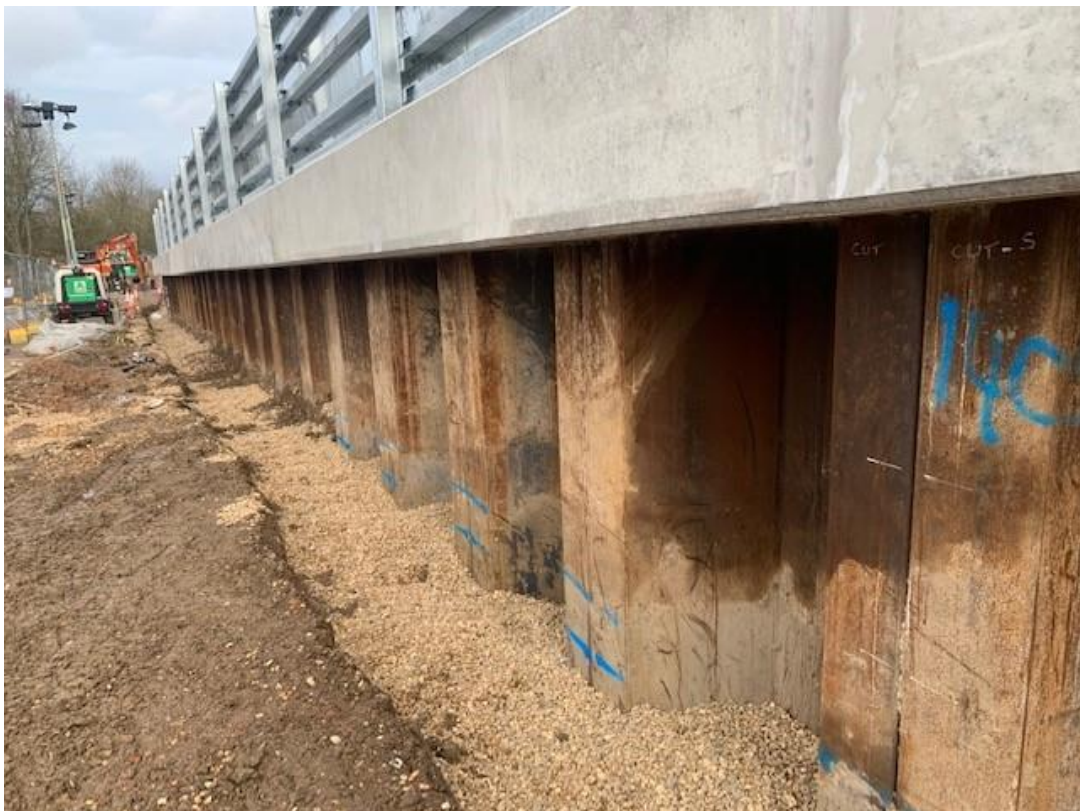
These pictures show the bare piled sheeting installed in position. The piles are 13metres depth with approx. 2 metres protruding above ground level.
